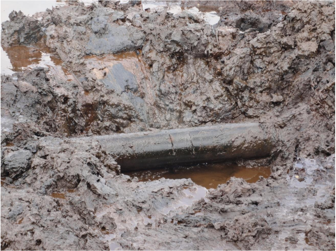
Overview: Hacksaw cuts visible on Well 13L flowline at Akaso. Picture was taken during JIV of 4 th May, 2011
