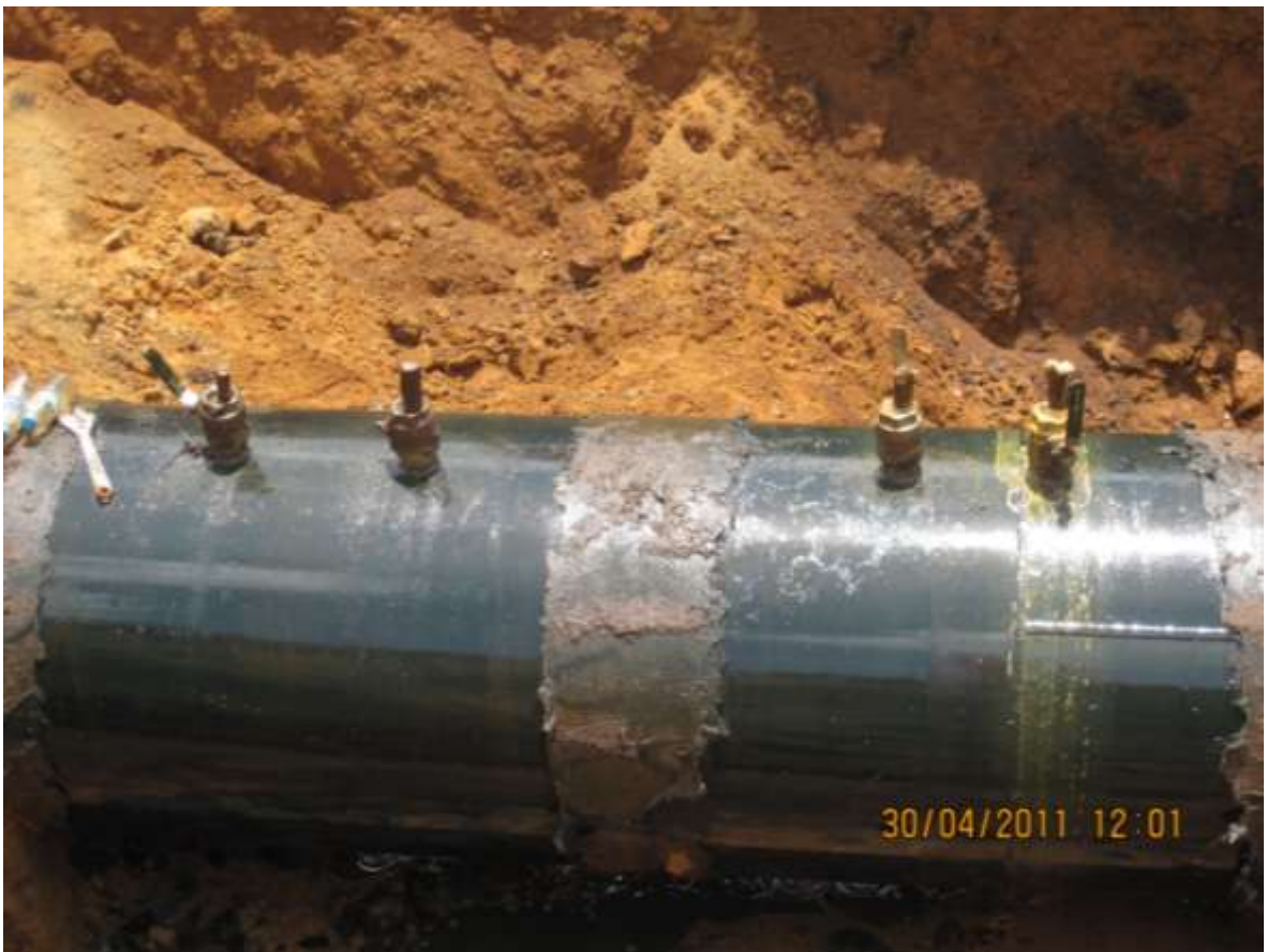
Close-up: Illegally welded points on 36'' Rumuekpe-Nkpoku Pipeline in Aluu. Picture was taken on 30 th April, 2011
