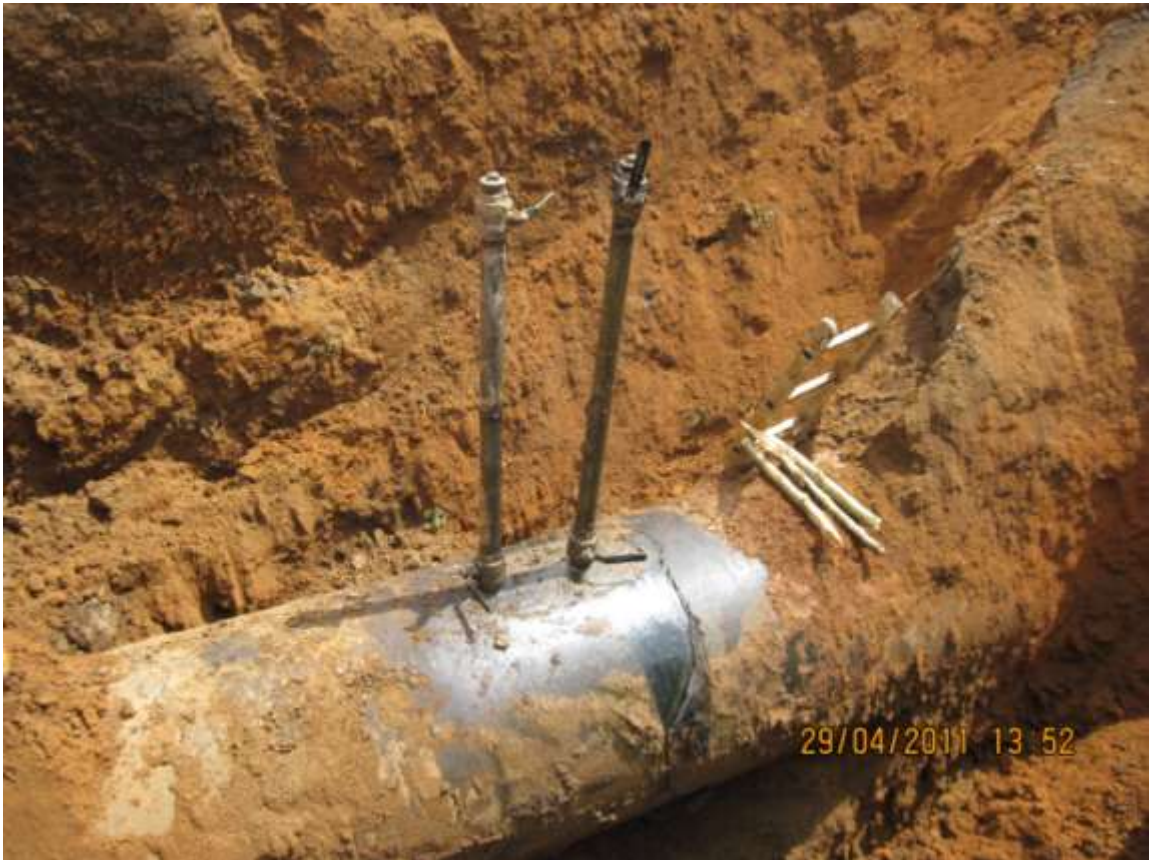
Overview: Illegally welded points on 36'' Rumuekpe-Nkpoku Pipeline in Aluu. Picture was taken during JIV of 29 th April, 2011
