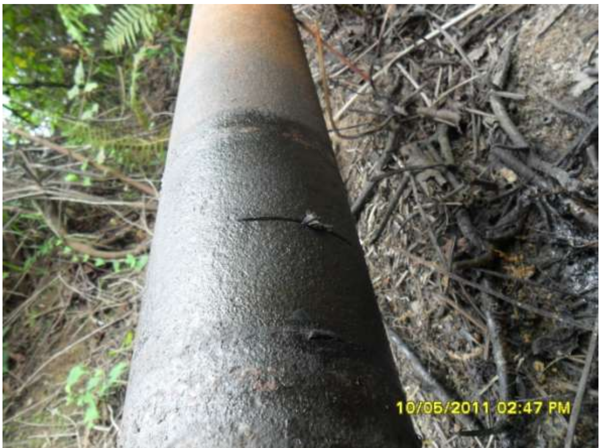
Close-up: Hacksaw cut on Oguta Well 17L flowline at Otuweneke-Umuayata. Picture was taken during JIV of 10 May 2011.
