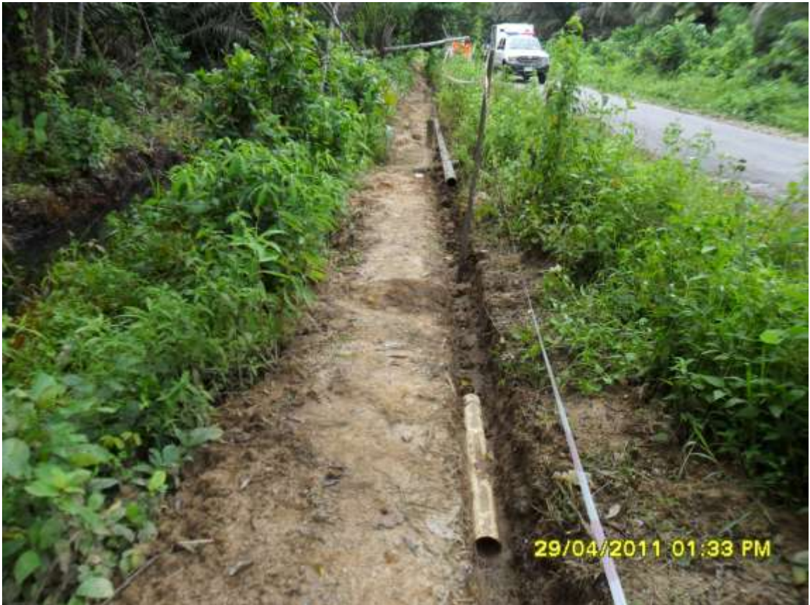
Overview: Missing section of flow line on Kolocreek well 21T flow line route in Kolocreek. Picture was taken during JIV of 29 th April, 2011
