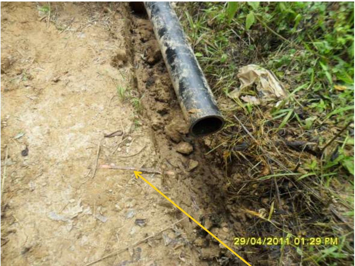
Close-up: Discarded used hacksaw blade can be seen beside cut section of flow line on Kolocreek well 21T.
