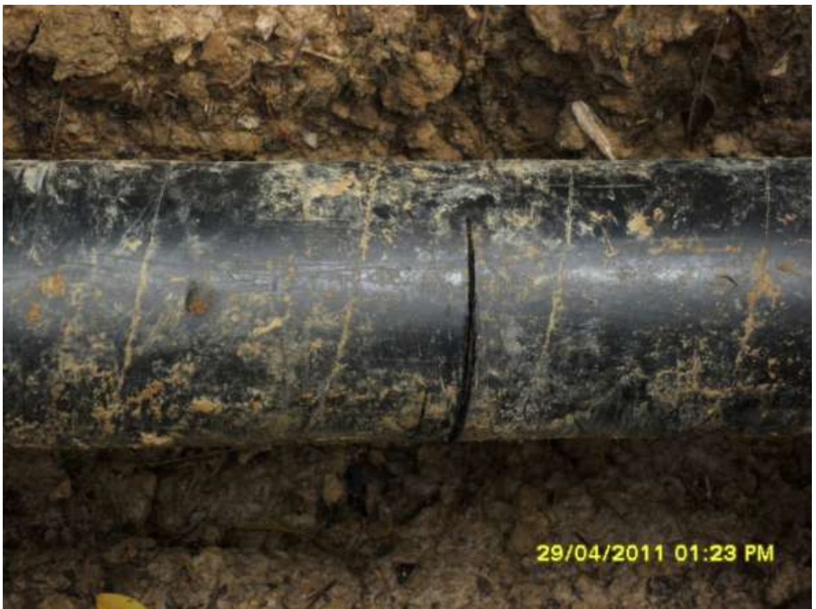
Close-up: Cut section of flow line on Kolocreek well 21T. Picture was taken during JIV of 29 th April, 2011
