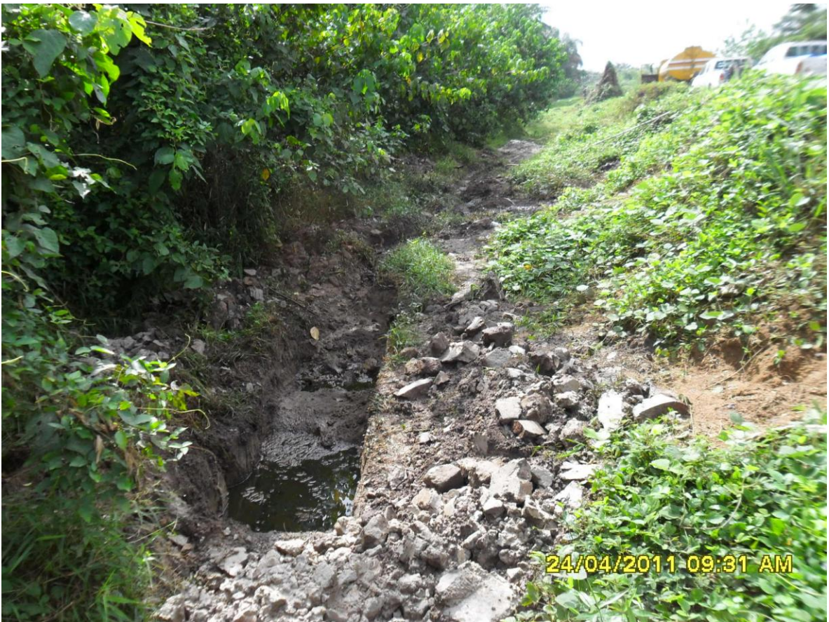
Overview: Extent of the spill incident impact at 12" Imo 2 – Ogale Pipeline route in Owaza . Picture was taken during JIV of 24 April 2011
