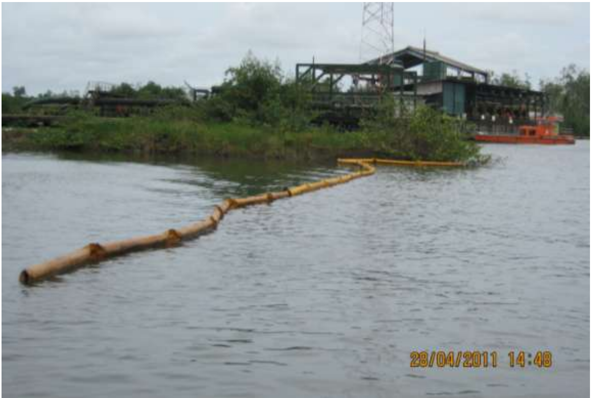
Overview: Partially removed Oil Boom placed around work area as a precautionary measure during replacement of the failed valve at Nembe creek 2 flow station.
