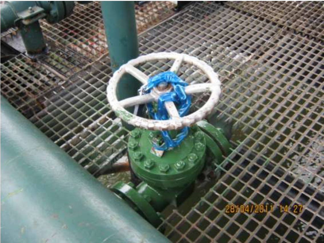
Overview: New valve replacing failed valve at Nembe creek 2 flow station. Picture was taken during JIV of 28 th April, 2011
