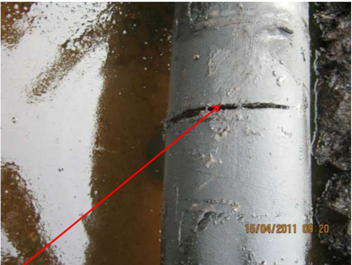
Close-up: Hacksaw cut on Akaso Well 3L Flowline route in Akaso. Picture was taken during JIV of 15 th April, 2011
