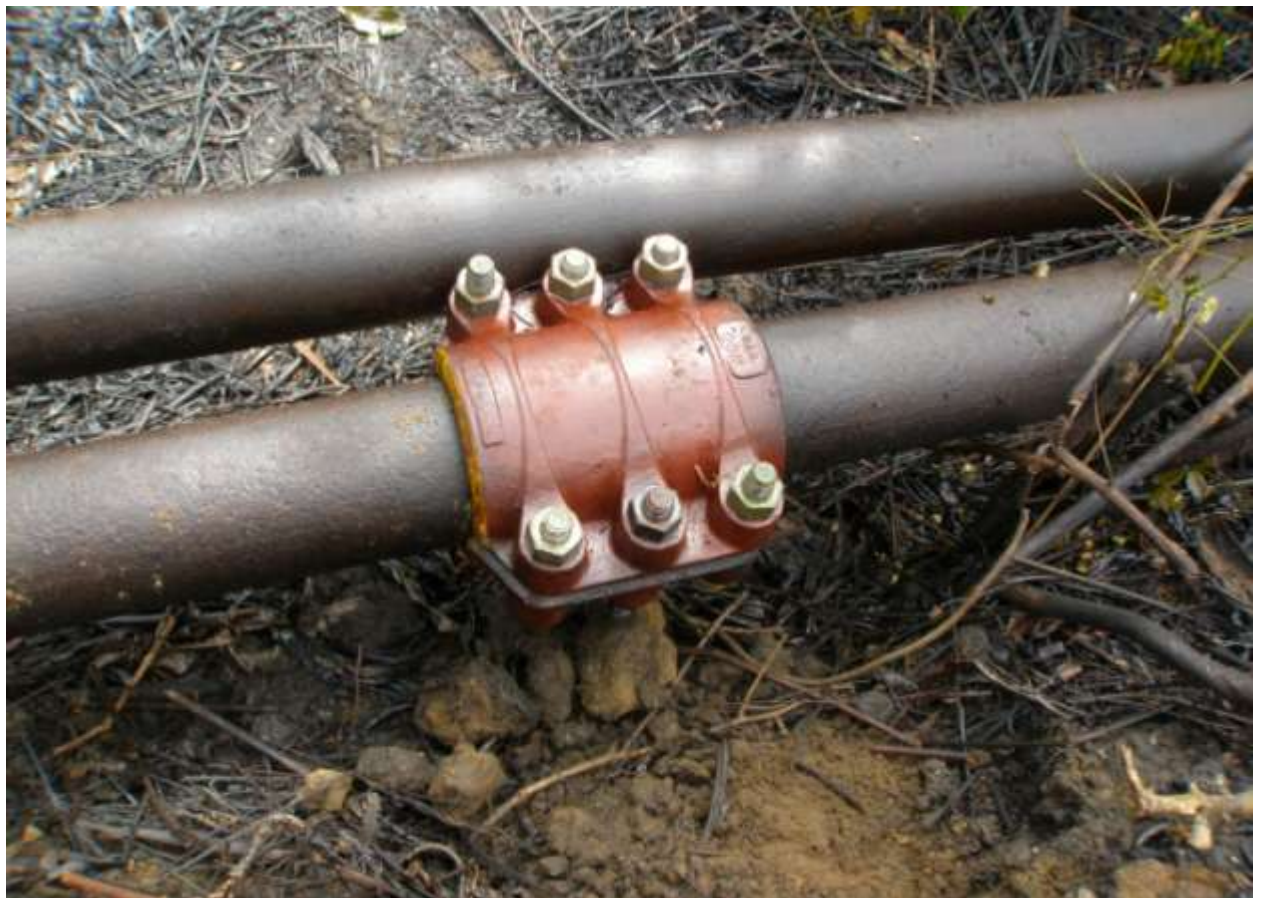
Close-up: Spill due to tampering with clamp nuts and bolts on Adibawa North-East Well 4L pipeline route at Biseni. Pictures taken during JIV of 11 th April, 2011.
