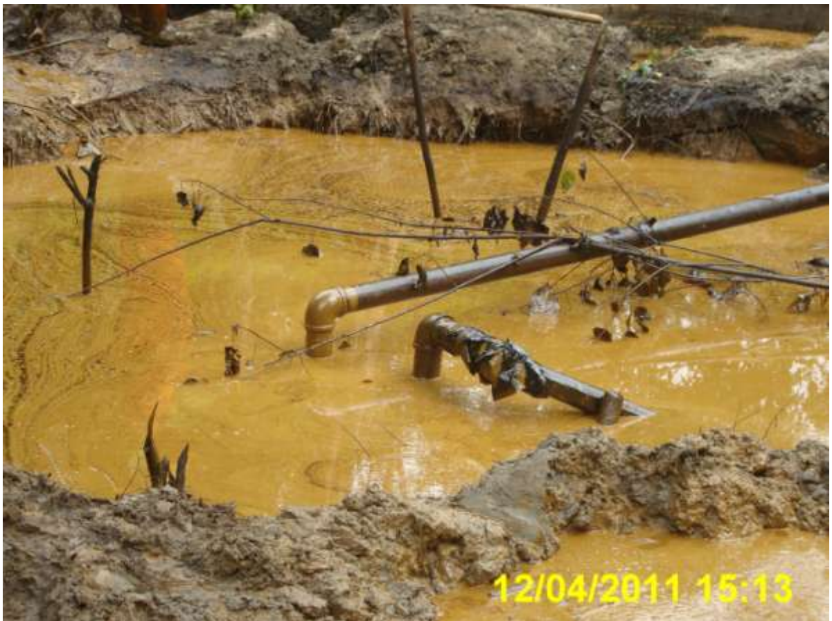
Close-up : Spill due to tampering on 8in Isimiri Pipeline at Umuaghala. Pictures taken during JIV of 12th April, 2011.
