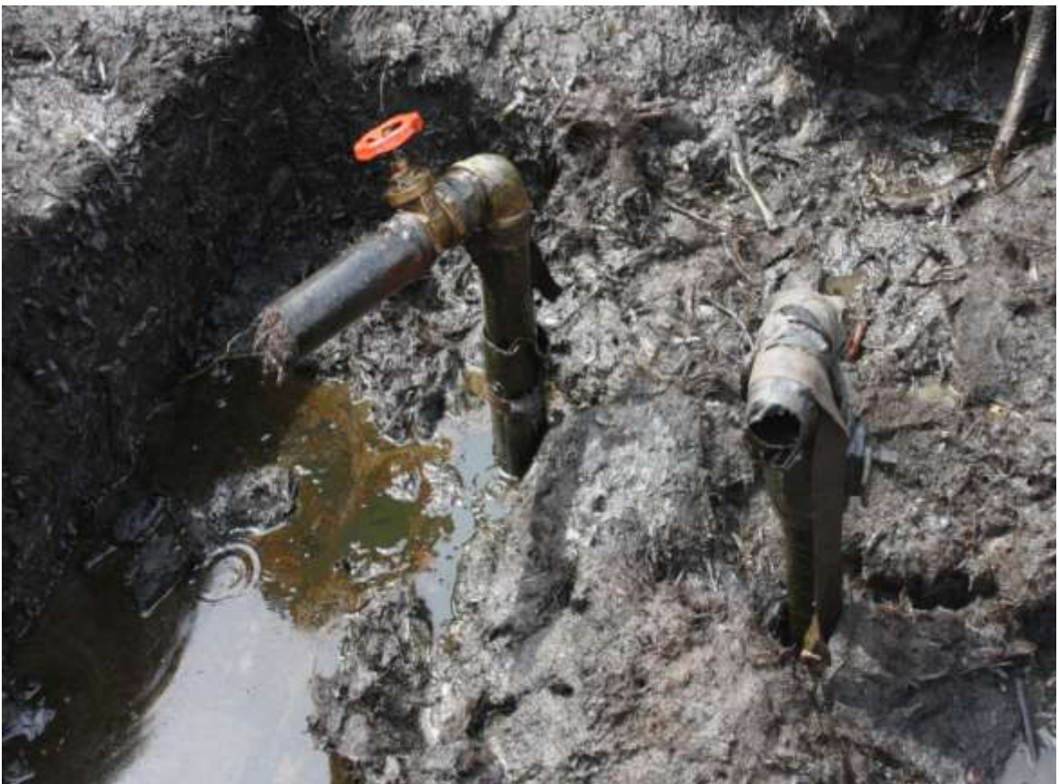
Close-up: Illegally welded points on 24" UPS-Rapele trukline at Ugbokodo. Picture taken during JIV of 6 th April, 2011.
