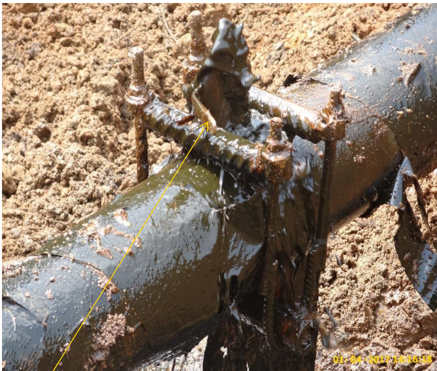
Close-up: Illegal fitting on 6" Obigbo North-Ogale Pipeline at Ogale. Picture was taken during Joint Investigation of 1 st April 2017.
