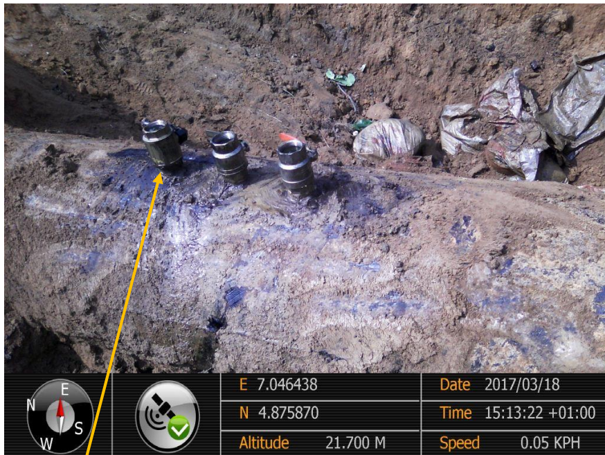
Close-up: Leaking Illegal fitting on 28" Nkpoku-Bomu Pipeline at Elimgbu. Picture was taken during Joint Investigation of 18 th March 2017.
