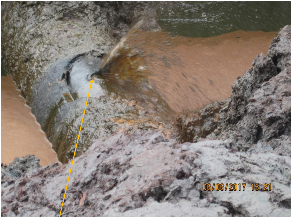
Close-up: Drilled Hole on 28" Bomu-Bonny Pipeline at Patrick Waterside. Picture was taken during Joint Investigation of 6 th June 2017.
