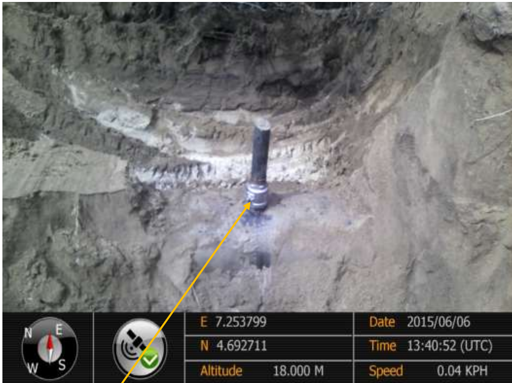
Close-up: Illegal fitting on 28" Nkpoku-Bomu Pipeline at B-Dere. Picture was taken during Joint Investigation of 6 th June 2015.
