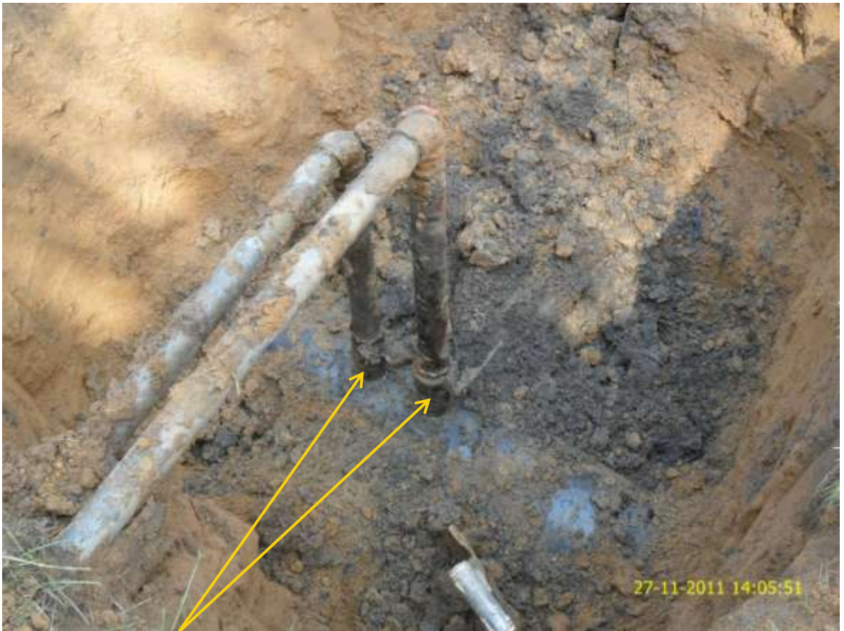
Close-up: Illegal fittings on 12" ImoRiver-Ogale pipeline at Owaza. Picture was taken during Joint Investigation of 27 th November, 2011.
