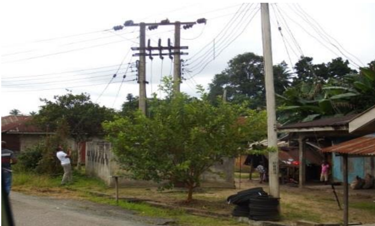
Plate 4.14h: Light Energy Transmitting Facilities
