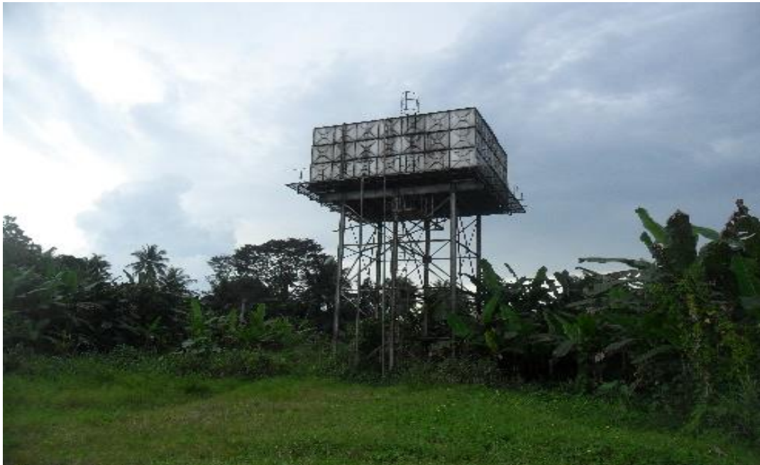
Plate 4.15d: Water facility in the Emughan communities
