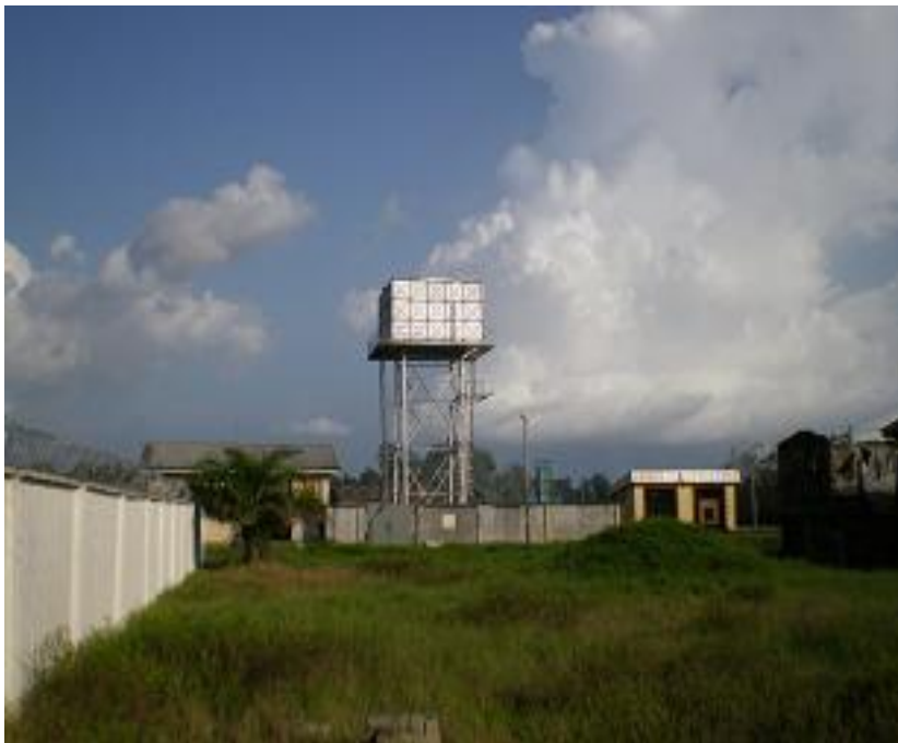
Plate 4.26: Water Borehole Facilities at Elem Sangama.
