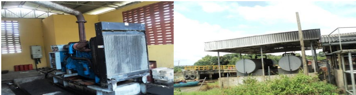
Plate 4.10.5: Two giant generators supplied by SPDC and DESOPADEC at Ugbeogungun community
