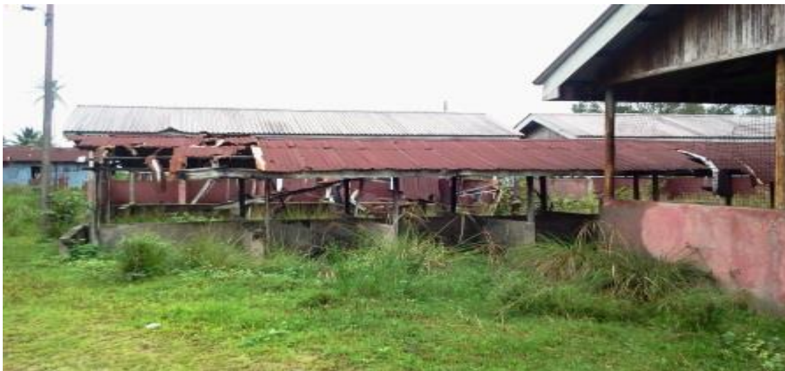
Plate 4.10.1: Destroyed market structures at Ugborodo
